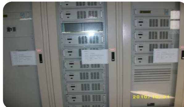
Charger Control System
